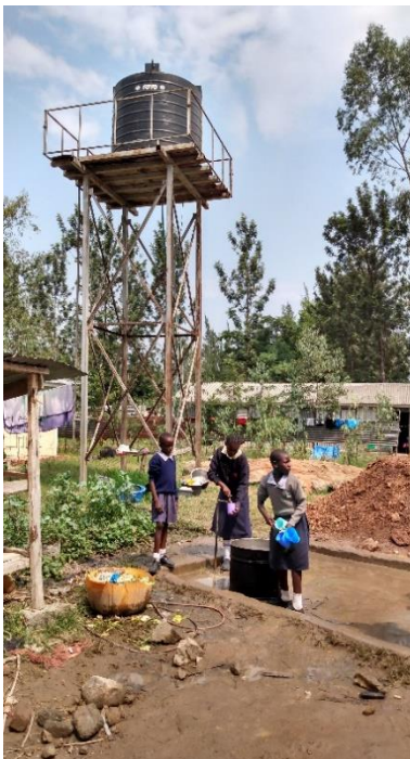
Water tower and pump
